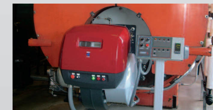
400 BHP Kewanee retrofitted with Riello Low NOx RS 400/BLU
